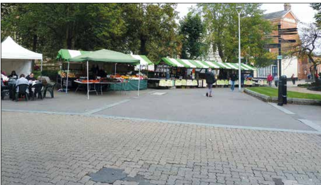
Patched block paving on Market Place
